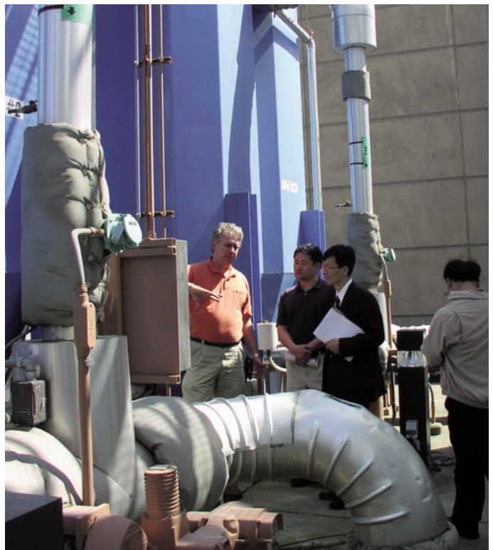
South Treatment Plant Reclaimed Water Facility
