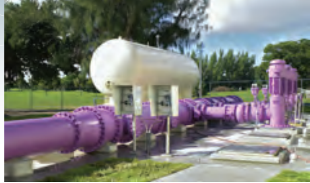
Pipes carrying reclaimed water
