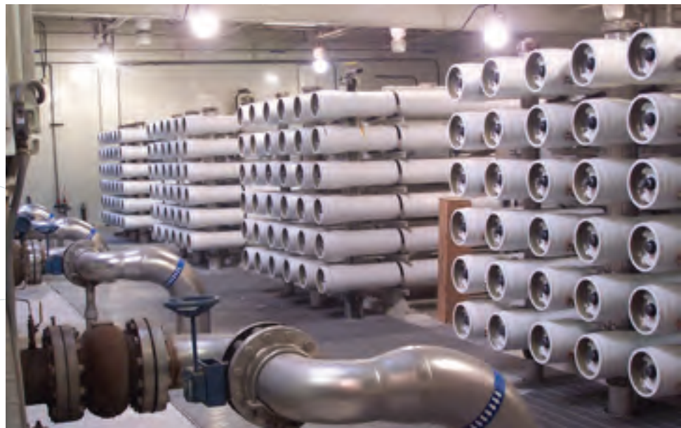
Desalters used to treat brackish groundwater in Chino, CA Photo courtesy of Inland Empire Utilities Agency
